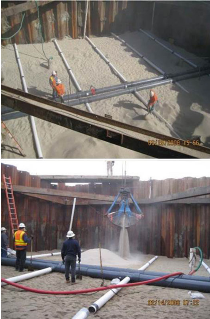
Fig. 11.14 Construction of the City of Long Beach test seabed gallery cell using sheet piling and dewatering the excavation prior to filter emplacement
