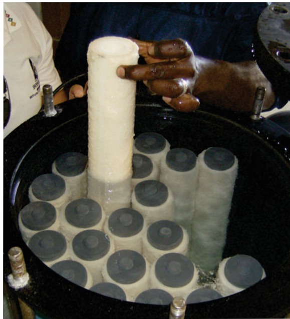
Fig. 8.1 Elemental sulfur coating the cartridge filters at a SWRO plant in the Bahamas. An air leak in the centrifugal pump caused mixing of the raw water containing hydrogen sulfide with air, causing the precipitation of elemental sulfur that caused shutdown of the plant
