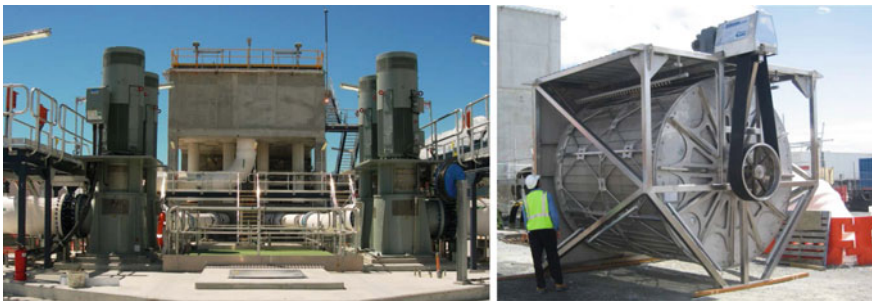
Fig. 2.8 Intake pumps and elevated screen structure 4 m diameter drum screen
