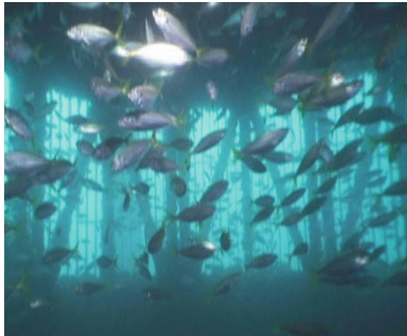
Fig. 3.15 View of the Gold Coast SWRO plant velocity-cap intake interior during operation
