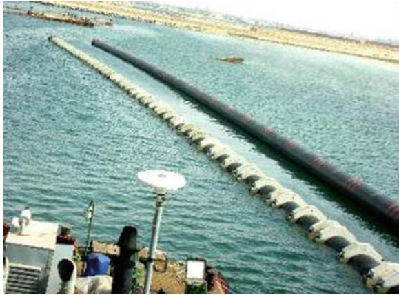
Fig. 5.11 Installation of conveyance pipeline for an intake system using the float, transport and sink method at Abutaraba, Libya
