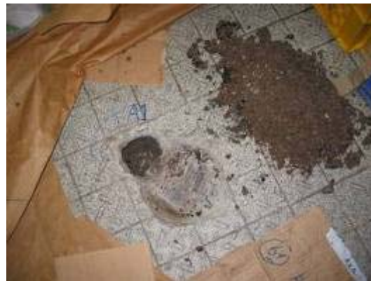
Asbestos insulation in floors underneath e.g. concrete
