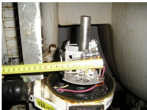
Figure 4: Typical level switch that may contain an ampoule with mercury
