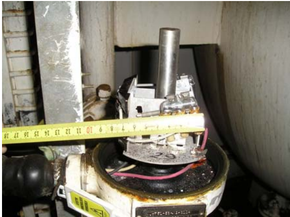
Typical level switch that may contain an ampoule of mercury
