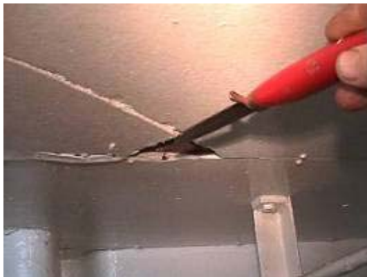
Asbestos in ceiling/wall plates and fire doors
