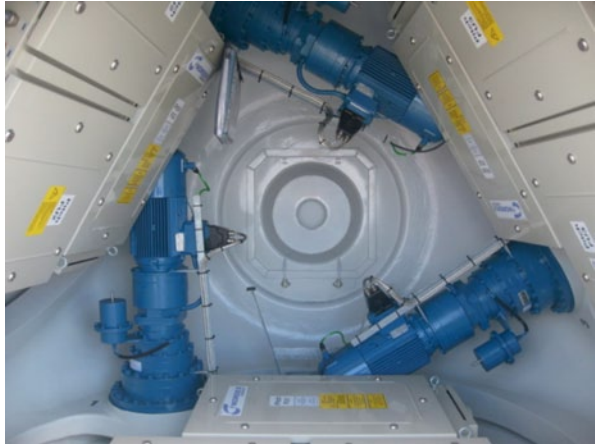
Fig. 2.6 Electric pitch system. (Courtesy of geograph.org.uk (Anderson, Interior of the hub of Turbine No 3, 2008b). © Copyright Paul Anderson and licensed for reuse under this Creative Commons Licence)
