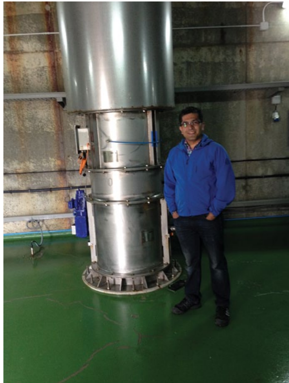
Fig. 5.6 Mutriku plant (300 kW). Author visit of the wave power plant in Spain. The picture shows a VOITH turbine with 18.5 kW installed power capacity
