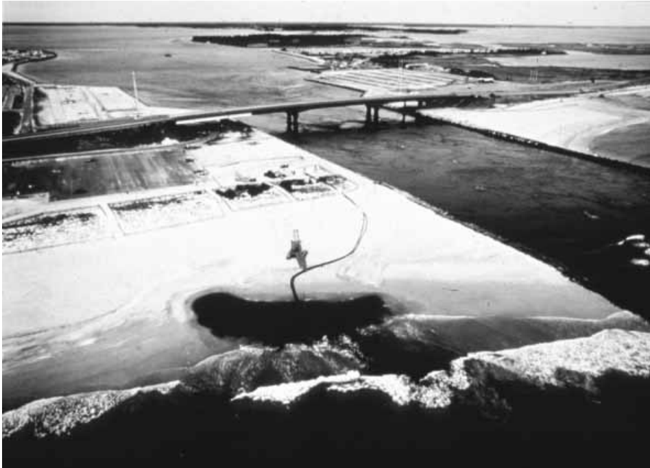
Figure 13.22 Indian River Inlet, Delaware, bypass system. The jet eductor pump is suspended from the crane and is lowered into the beachface, forming a temporary excavation crater.
